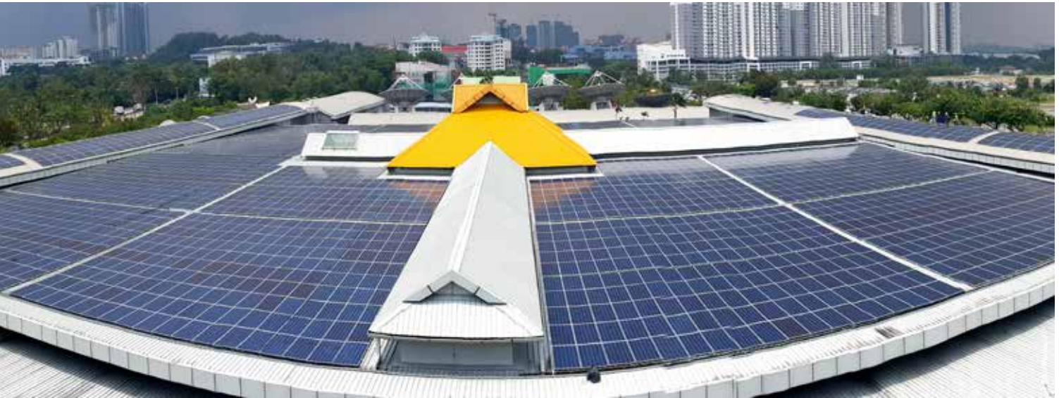
We installed more than 4,700 solar panels at Astro headquarters with the ability to generate 1.8 million kWh of electricity per annum
